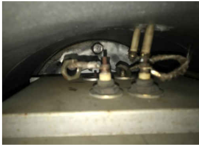
Figure 65: Wiring issue with autoclave
